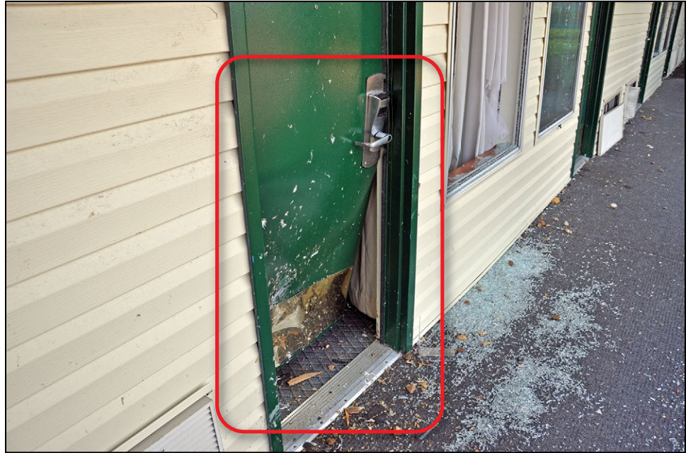
Figure B8-23. This metal door was damaged by wind-borne debris generated by a weak tornado. The bottom hinge was damaged, but the single latch was able to resist the modest wind and impact load. The door was on the verge of failing. (St. Louis, MO, 2013 tornado)
