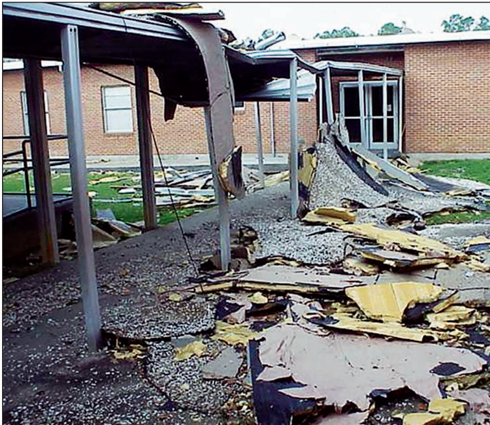
Figure B8-2. Medium debris: Pieces of a built-up roof from Hurricane Katrina (MS, 2005)
